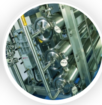
Process water systems
